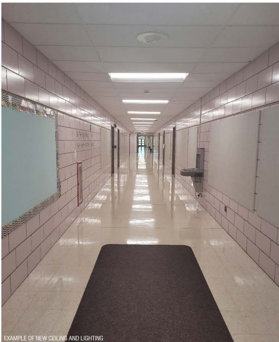
EXAMPLE OF NEW CEILING AND LIGHTING
